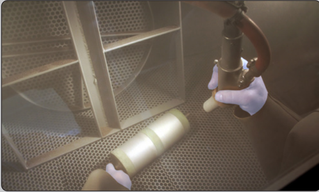
A cylinder masked with 170-10s (Green) Masking Tape is undergoing grit blast prior to receiving thermal spray coating.
